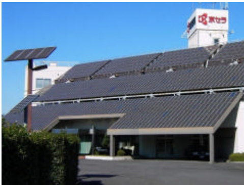
43kW system installed at the Kyocera Sakura Solar Energy Center
